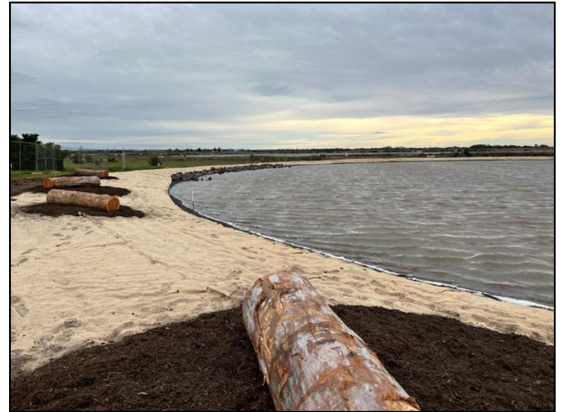
Plate 2. Large logs placed atop mulch piles along wetland edge (Ecology and Heritage Partners 15/08/2025)
